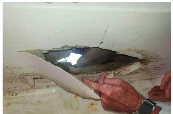
ABOVE: The problem hole.
